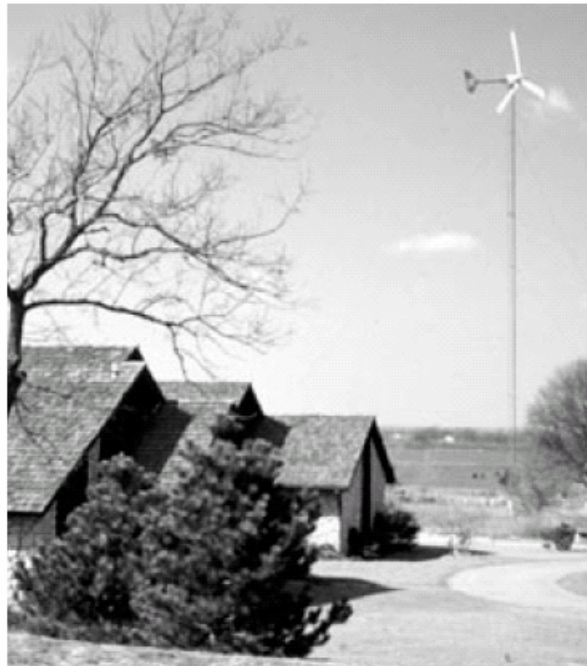
Homeowners, ranchers, and small businesses can use wind-generated electricity to reduce their utility bills. This grid-connected system installed for a home in Norman, Oklahoma, reduces the homeowner's utility bill by $100 per month.
